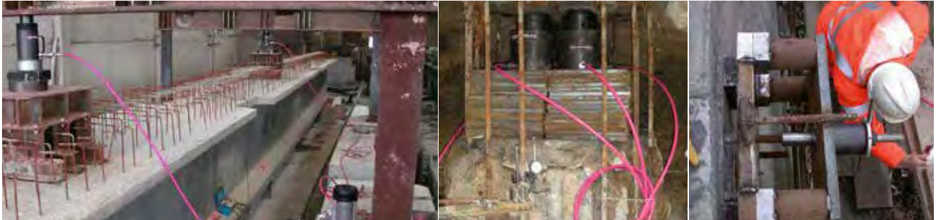
Deflection test on prestressed beams with Europress big tonnage cylinders and power packs.
