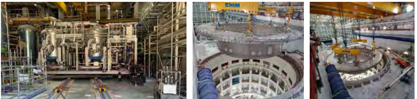
Numerous special EUROPRESS cylinders and power packs have been vital for the operations of shifting and correct positioning of the structural parts of the Tokamak, the beating heart of the ITER reactor. San Paul Les Durance, France.
