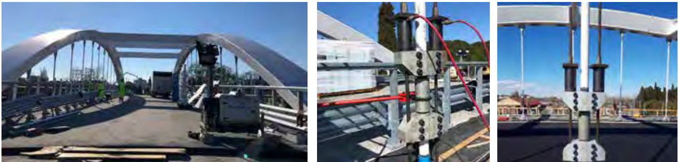
CMF hollow cylinders and double stage PN hand pumps for the positioning of the deck and of the tie-rods which tie the latter to the arches of the new "Ponte Teodorico". Ravenna, Italy.
