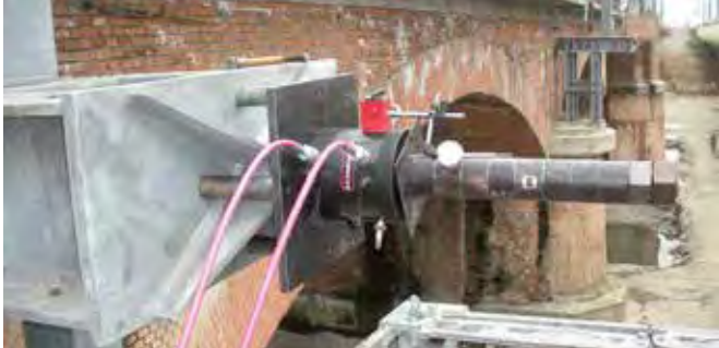
COF Hollow ram cylinders for anchor bars stringing on a railway bridge.
