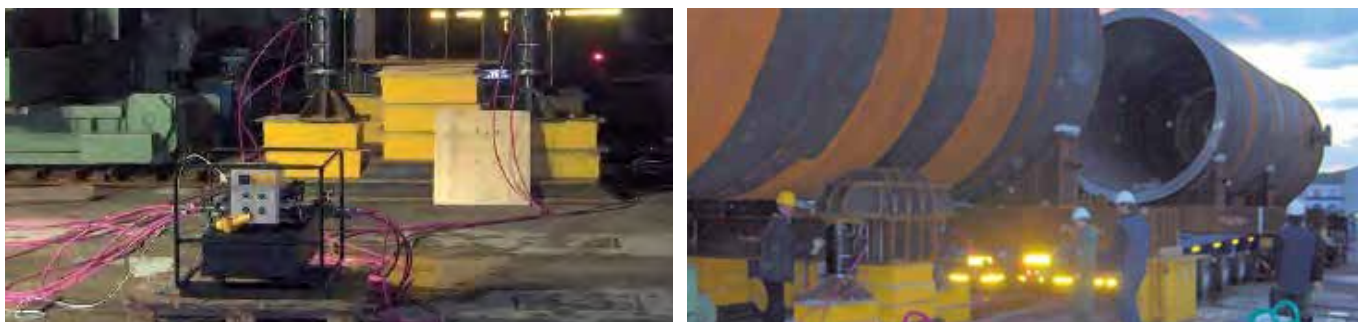
Lifting of the shell of the container for the construction of a reactor destined to the oil sector. The cylinders are operated by a Split Flow Power pack.
