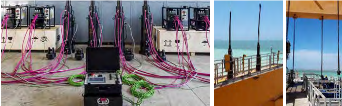
Strand jack system for the synchronized lifting of heavy loads by using metal cables.
