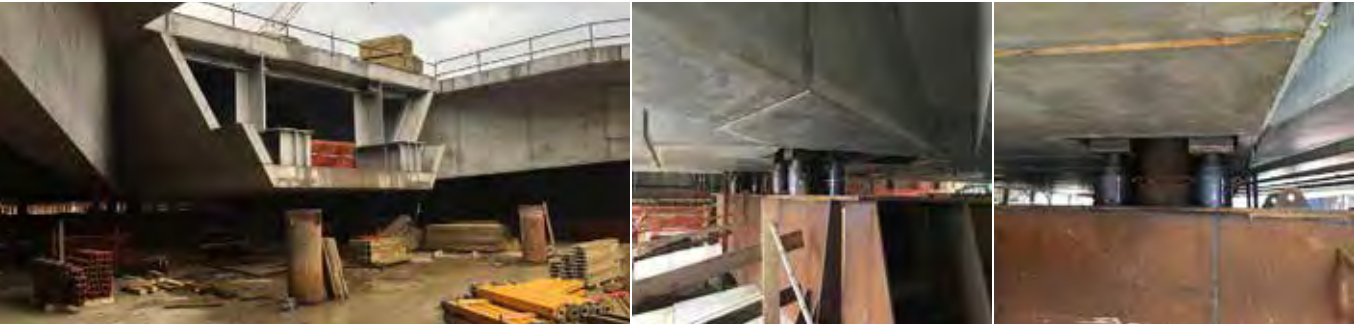
Positioning of the roof insole in the new high speed Belfiore station with the help of ME power packs and CGG cylinders. Florence, Italy.
