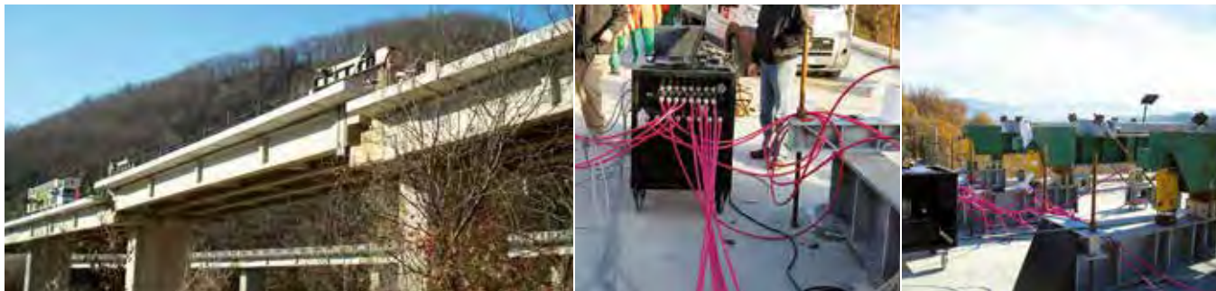
Synchronized lifting system on the Piacenza Brescia motorway viaduct for the substitution of the anti-vibration supports. Ponte Sarmato, Italy.
